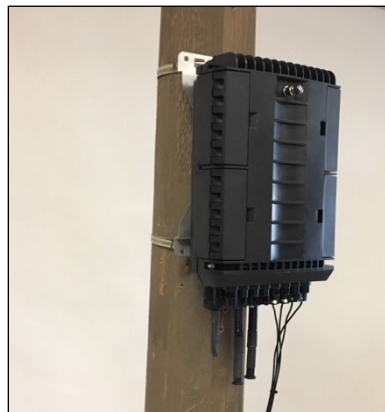
Figure 11 Pole Mounted FSDC-G
