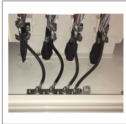
Figure 7 Cable Attachment Hardware Connected to Ground Bar
