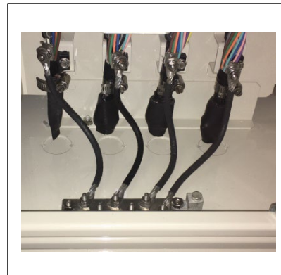
Figure 9 Cable Attachment Hardware Connected to Ground Bar
