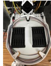
Route Fibers in the Splice Tray
