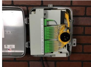
Distribution Cables Connected to Bulkhead
