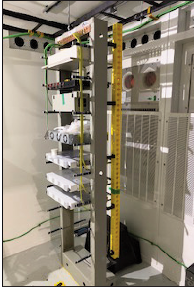
Interior View - Ericsson Racks
