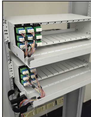
CPRI Monitoring Rackmount Shelves
