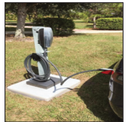
• Electric Vehicle Charging Stations
