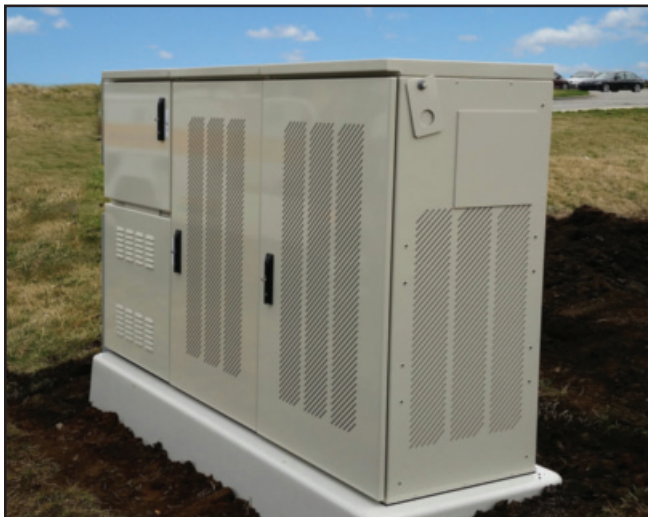
3-Bay CPAD installation with CUBE High-Power Small Cell Cabinet
