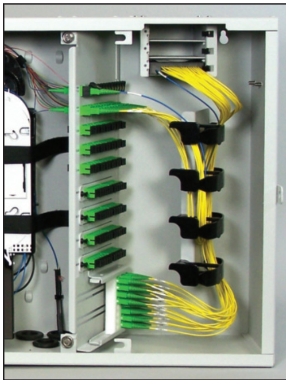
Charles Fiber Splitter Module (CFSM-FM) in a Charles Fiber Building Terminal (CFBT).
